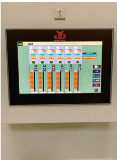
JB Machinery Control Panel
